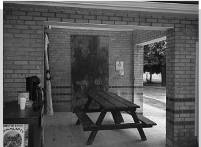
Women's Washroom Door - Not Ready Yet
